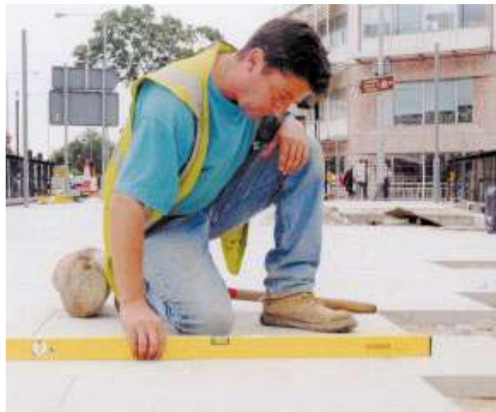
Improving the footway with high quality surfaces – laying York stone paving in London.
