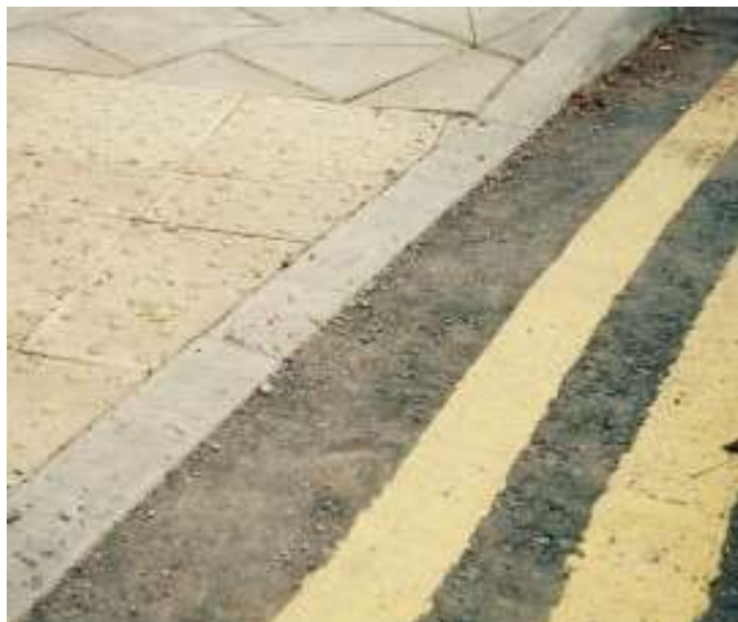
Fully flush kerbs are desirable, so long as drainage is adequate. Courtesy: Tony Russell.
